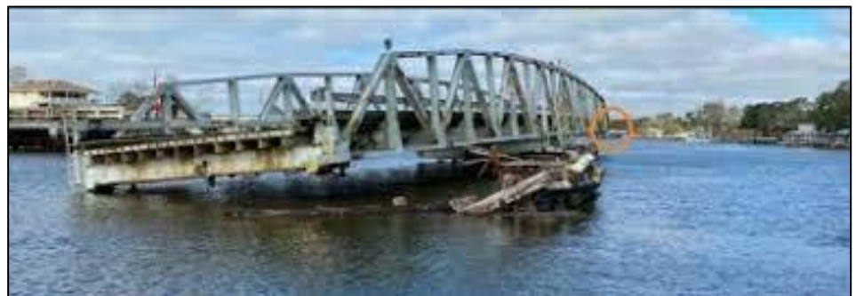
Tow accident with the Centerville Bridge. Image workboat.com
